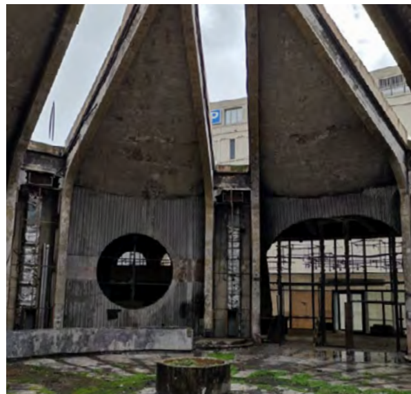
A major fire in 2013 severely damaged the dome and the hall's interior; since then, the building has fallen into disrepair
